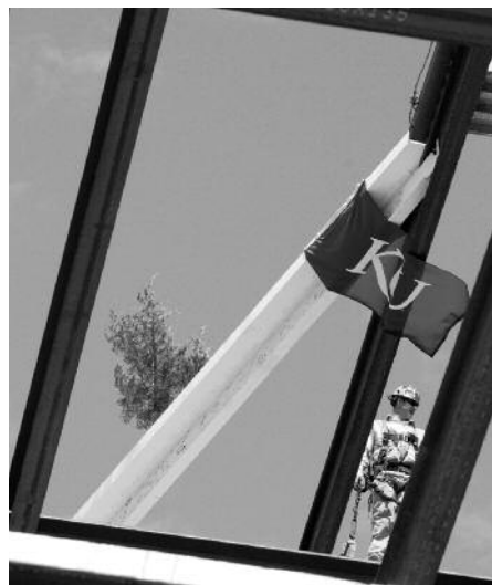
Signed and decorated with flags and a good luck tree – as is construction tradition – the topping-out beam was put into place atop the six-story structure.
